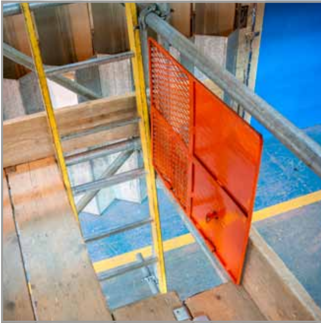
Ladder Safety Hatch - Open Position
